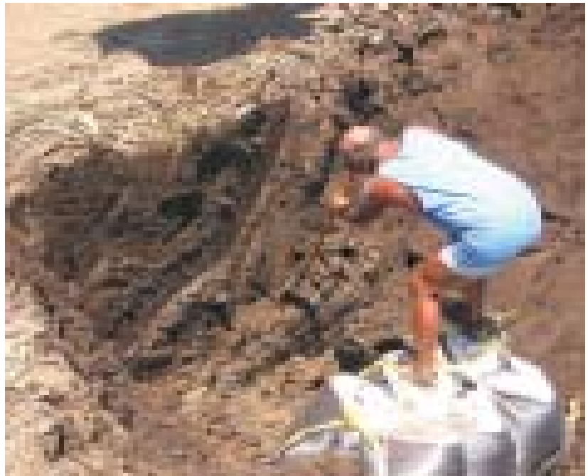
Alan Harn excavating from atop saddle bag anchors over pipeline. Photograph by Sally McClure.
