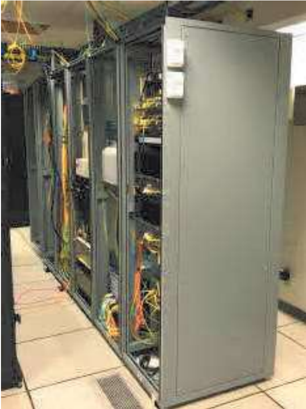
Technology Equipment at HSB
