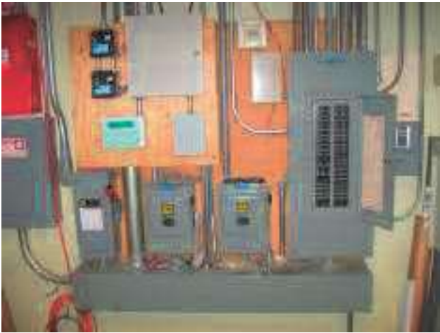
Electrical Equipment at Legacy Campus
