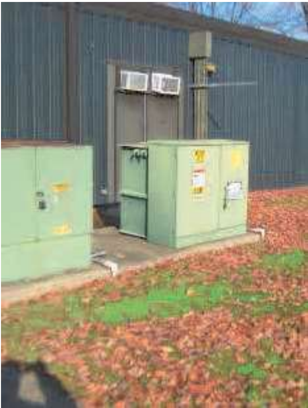
Electrical Equipment at Legacy Campus
