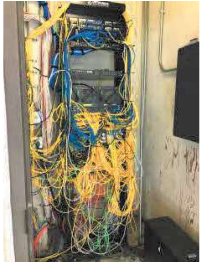
Technology Equipment at Brookens Library
